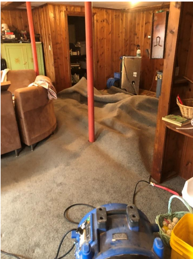
This technique is called “floating” the carpet, done AFTER removing soggy carpet pad that has no chance of responding to any drying techniques – only specially designed carpet pad can be dried, and even then, not always.
