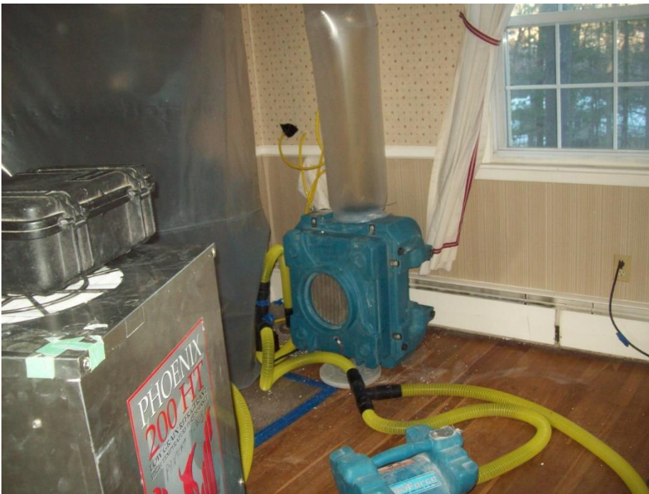
Sometimes the setups are much more complicated – like when there is accumulated water in the ceiling and the walls, plus on and under the hardwood. This type of a situation could occur as a result of a hurricane or when there are ice dams, like this New England loss.
