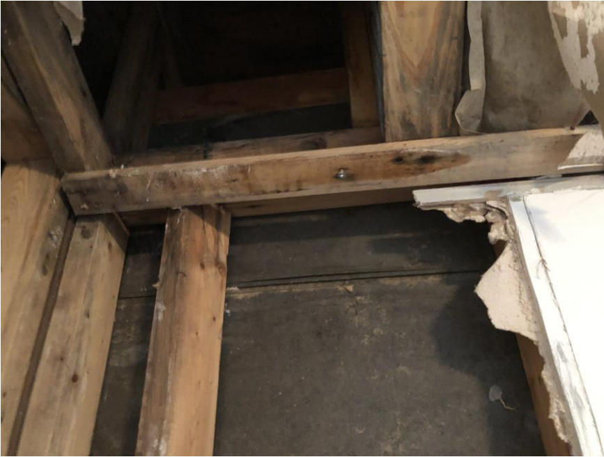
Furring for wall board is stained and wet in this area. 2/27/2021. Ambient drying will occur here. Snow is melted from roof top, and a tarp set up by the association was placed.
