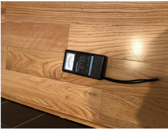
Water under engineered floor in front of fireplace 2/22
