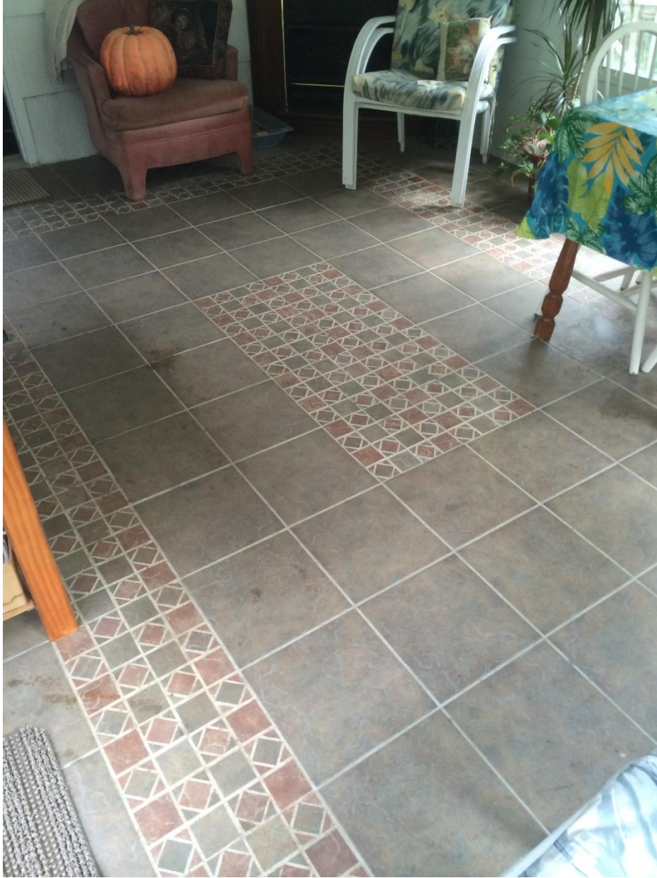
THIS IS A FOUR SEASON SUNROOM/LANAI WITH CUSTOM INLAY AND BORDER USING A NON-SLIP 12x12 TILE
