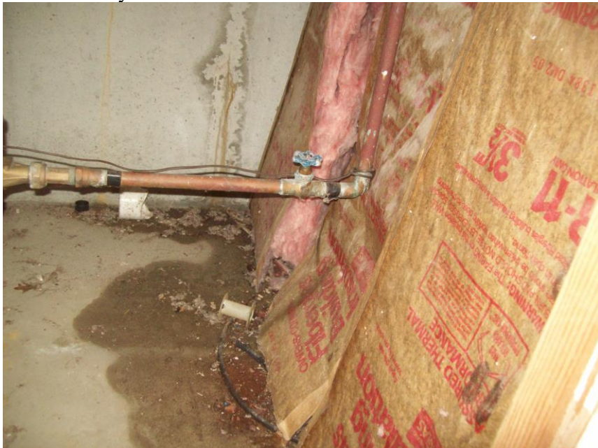
11) Behind basement closet below stairs, whole house shutoff area
