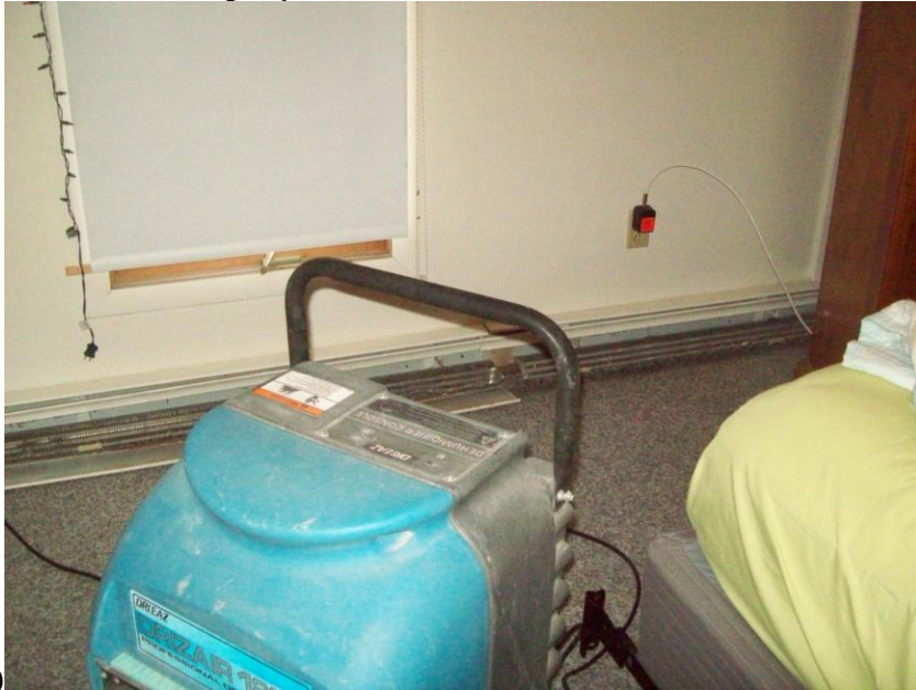
1) Pipe break in first floor bedroom near the electric service panel.
