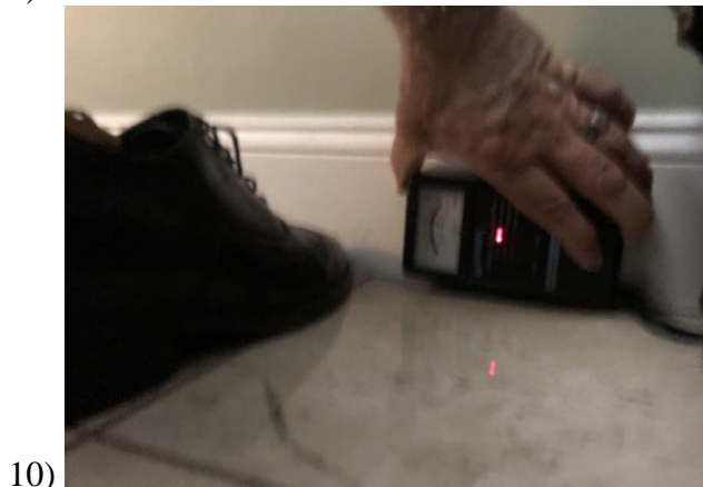
Master Bedroom closet thermal images and areas impacted by water damage. J-Peg images 7 and 9 are the air handler tray still loaded with water
