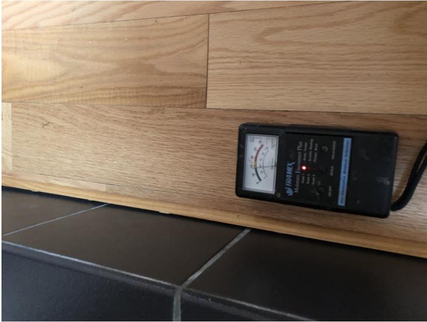
2/27/2021 – Removed dehu and floor drying equipment with normal wood material moisture content typical in New England in winter months.
