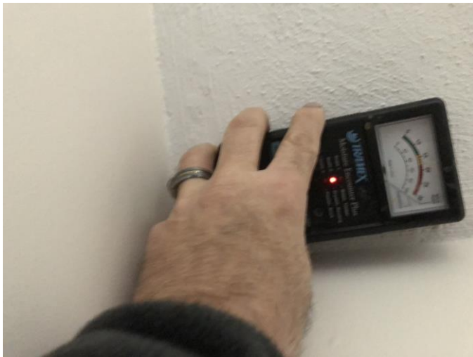
Water in ceiling 2/20
