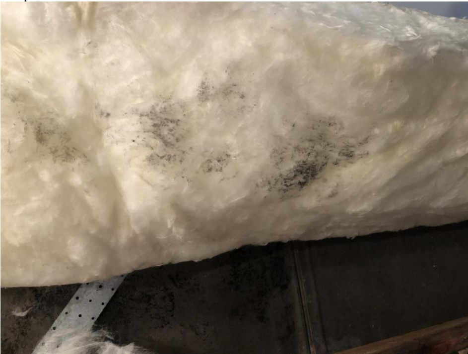
Suspected mold colonies on the back of the insulation
