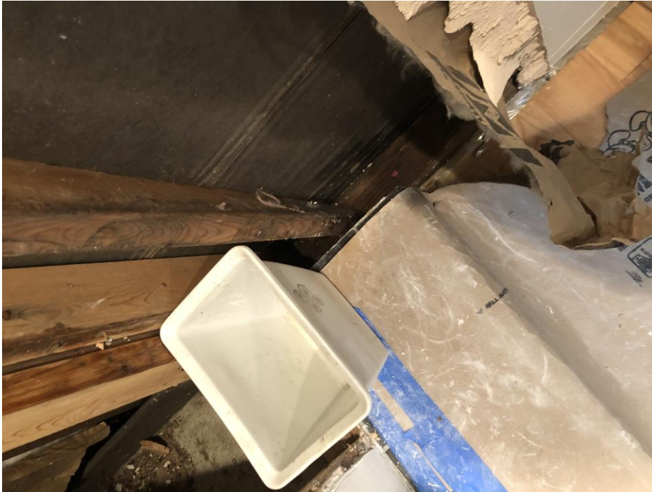
Water falling from ceiling into receptacle – 2/22/2021
