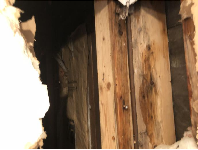
Active water photographed upon opening wall bays to the right of the chimney chase
