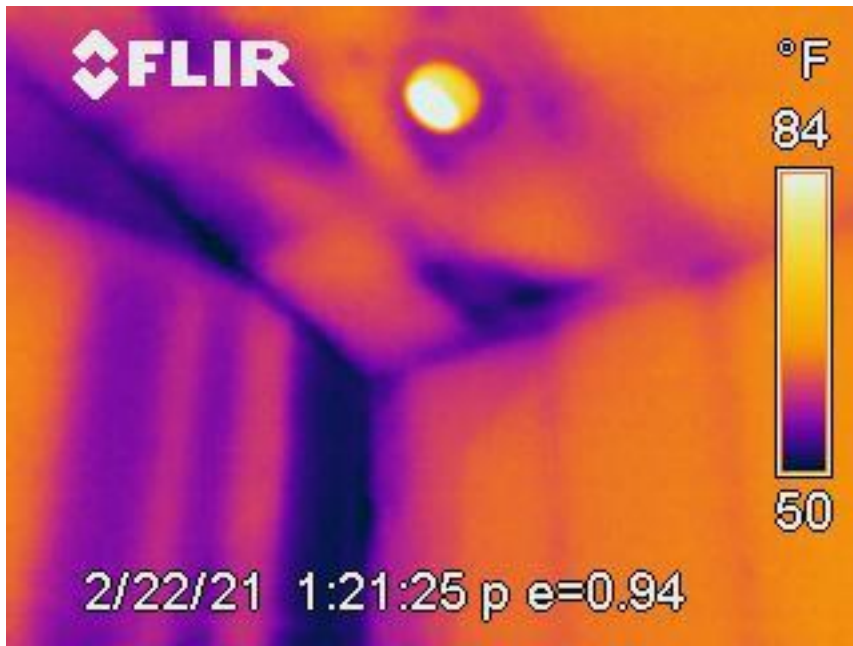
Water accumulation at the bottom of the ceiling slope and in the affected wall bays as shown.
