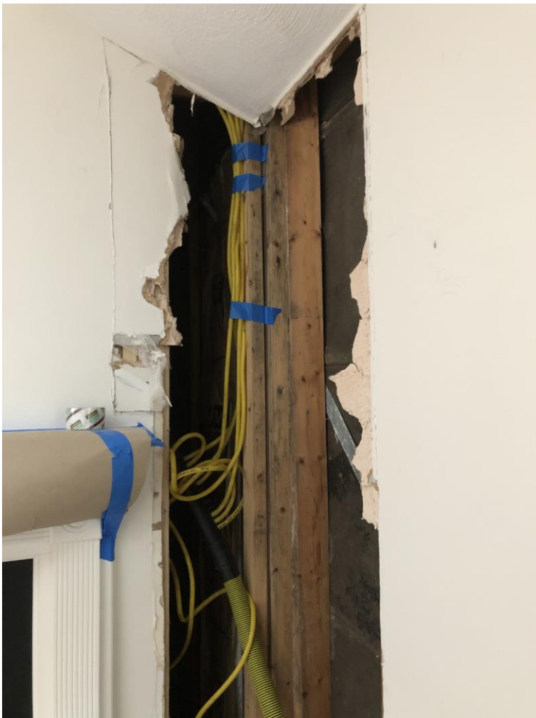
Monitoring visit #3 2/24. Re-assembled DriForce InterAir system to blow warm air into stitial space in ceiling cavity -did not wish to disseminate suspected mold (await sample results from CEI Labs)
