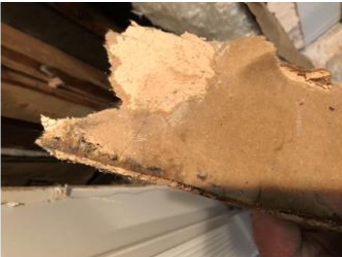
Some suspect mold presence on drywall
