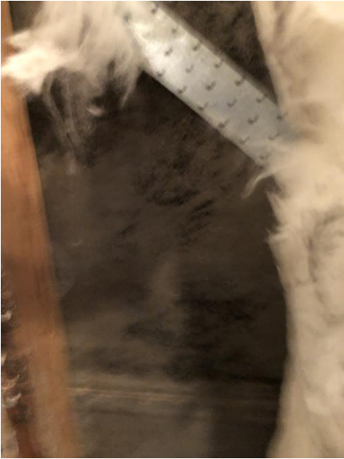
Suspected mold on insulation and the back of stucco
