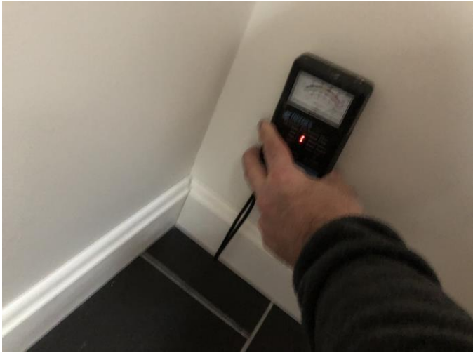
Water in wall bays on rear wall of great room 2/20
