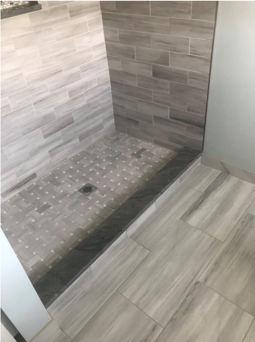
KBRS, TEC and Laticrete products with a custom granite dam were used here, and a brushed nickel tile edge give it the modern look the owner wanted.
